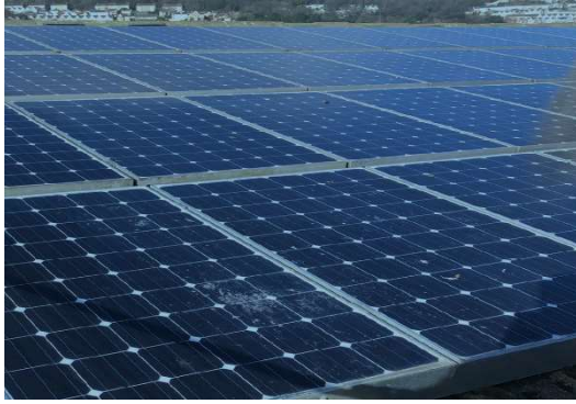
Solar PV modules installed on the Guildhall
